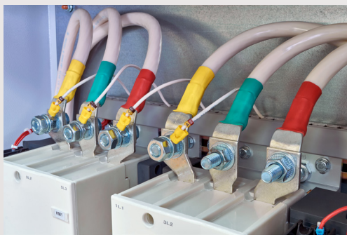
Contact cleaner should be able to be sprayed on energized electrical circuits without concern.
