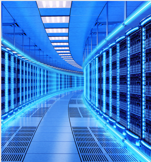
Large scale data centers typically house millions of servers connected by hundreds of thousands of feet of fiber optic cable.
